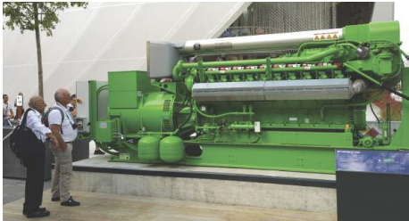
GE's Jenbacher Gas Engine behind the US Pavilion
