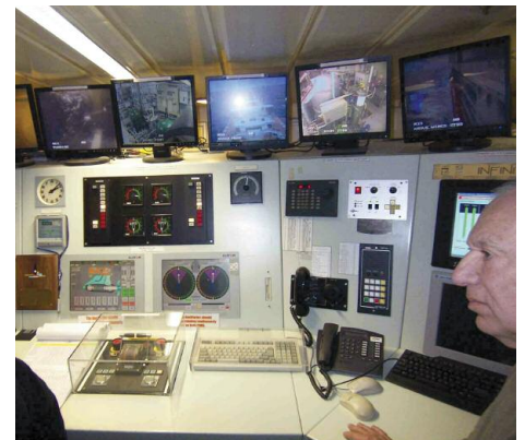
Engine Control Room of the Celebrity Infinity
